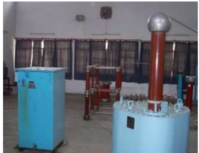
Voltage regulator and high voltage transformer
